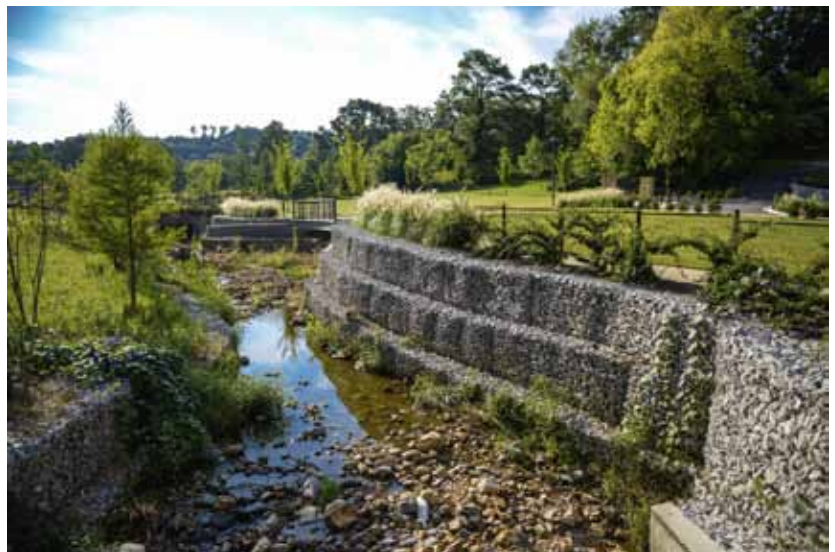
Crestwood Park - Restored tributary of Village Creek with Gabion walls. Photo © Abraham Odrezin; used with permission.
